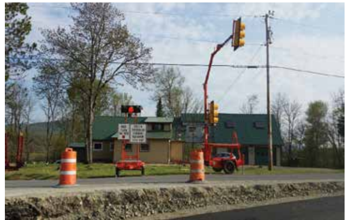
Figure 60. DAD and Temporary Traffic Signal (Courtesy of Horizon Signal 35 )
