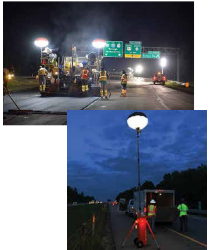
Figure 57. Task Lighting and Presence Lighting (Courtesy of NCDOT)
